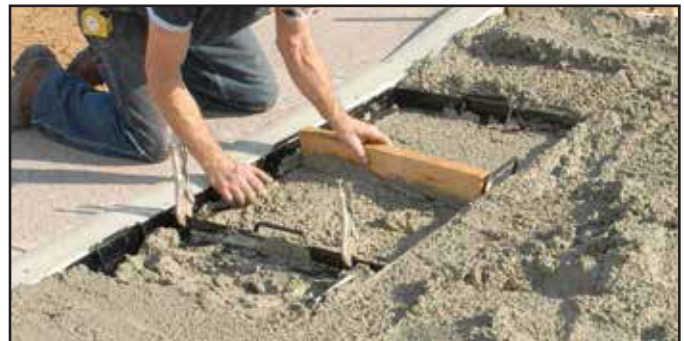
6) Level concrete with a straight edge inside of the frame work- adding concrete as needed. Note: Standard frame designed for 2" thick paver.
