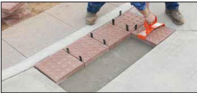
Step #3 - Thin Set Installation - Set pavers. Be sure pavers are fully set into thinset. (Back buttering may be necessary).
