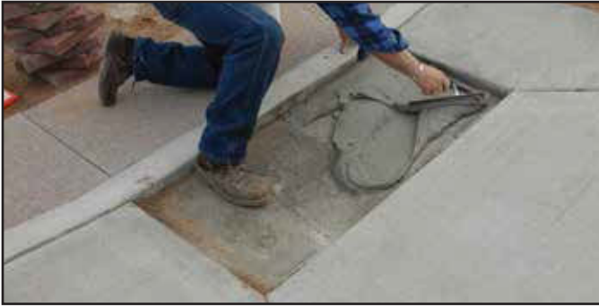
Step #1 - Thin Set Installation - Apply thin set with 1/4" x 3/8" notched trowel. Exterior grade.
