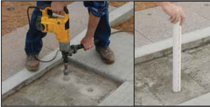
Step #1 - Sand Set Installation - Create weep holes for drainage. Core drill hole once concrete has set or, while concrete is still wet, make a hole with pipe.
