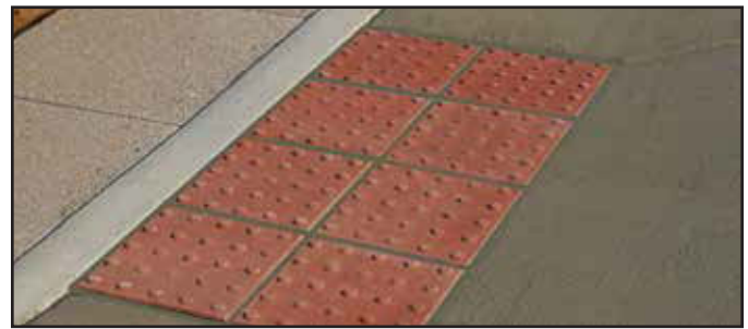
Step #4 - Thin Set Installation - Grout all joints with an exterior based grout or caulk. Complete.
