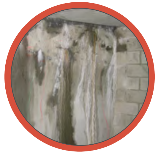
Classic example of a failed waterproofing system
